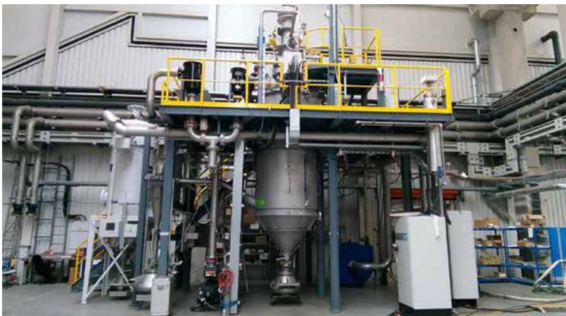
Amaero will expand its metal powder production capacity with the addition of a fourth atomiser (Courtesy Amaero)
