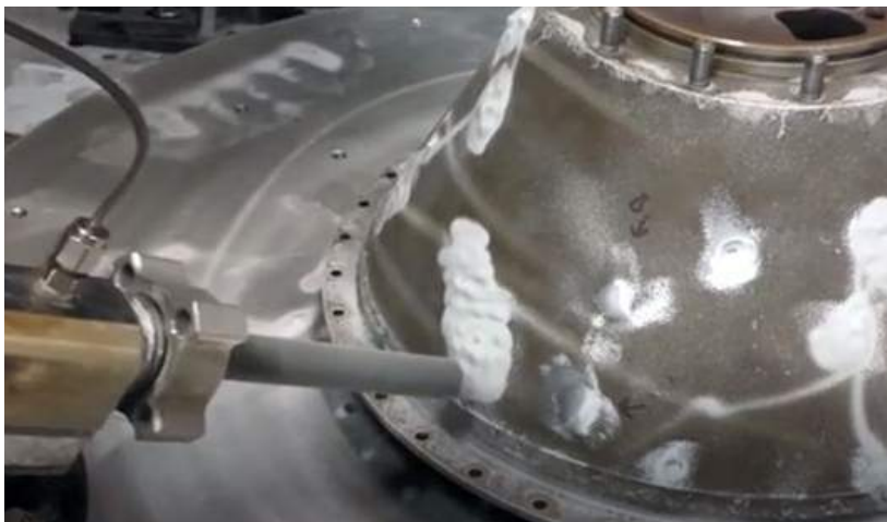
Cold spray Additive Manufacturing can be used to perform surface repairs on damaged metal structures (Courtesy Worcester Polytechnic Institute)
