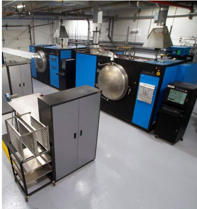
Fig. 3 This view of the DSH facility illustrates how additional facilities required to run a furnace, such as process gas supply, air, power, water cooling systems, etc., involve expenses that can often go unrealised in an analysis
