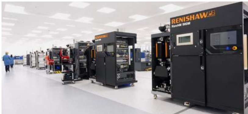
Renishaw is planning to co-locate its AM technical and commercial teams in its Gloucestershire facilities (Courtesy Renishaw)
