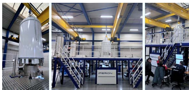
IperionX's HAMR furnace in the Titanium Production Facility (Courtesy IperionX)
